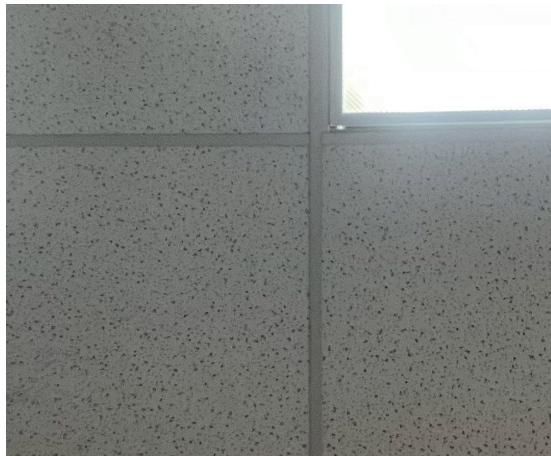
Figure 3. Photo of the Author's Office Ceiling (2022)
