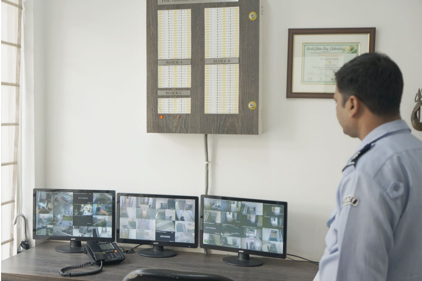
Figure 6: CCTV at The Golden Estate, 2014, Faridabad.
